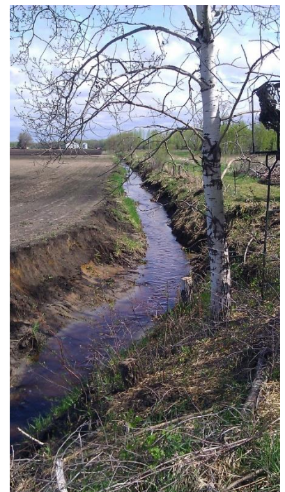
Example of drainage system that would benefit from stabilization practices.
